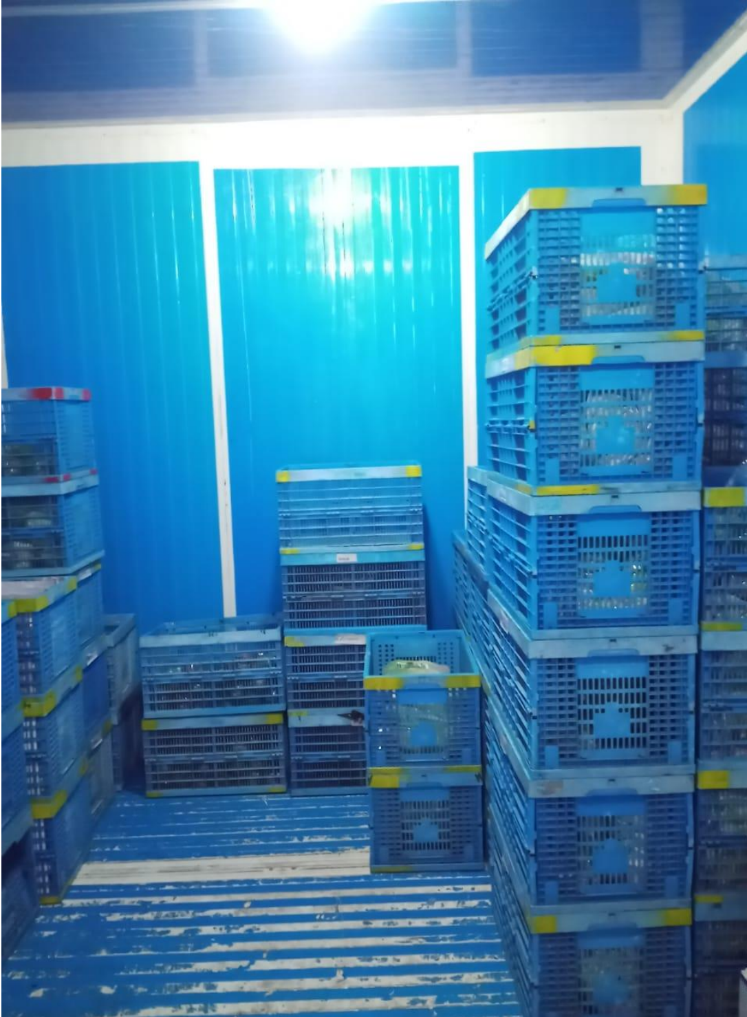
Lampiran 1 Ruang Chiller
